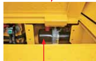
Pump and motor
