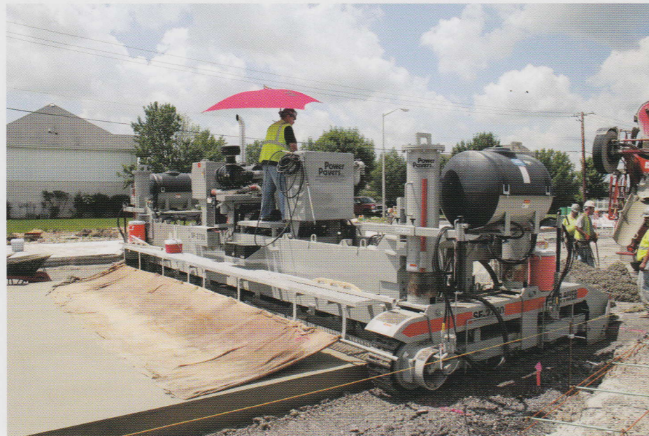
SF-2700 paving a street. Hooks for a burlap drag are standard on the rear catwalk.
