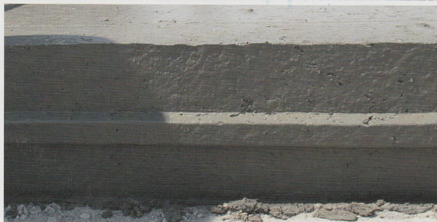
Edge of pavement with optional key-way inserter (top), and optional male key-way block-out (bottom).
